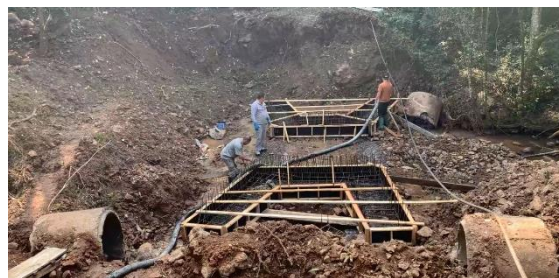
New Bridge Construction (The previous bridge on our property was destroyed during last quarter's storms)
